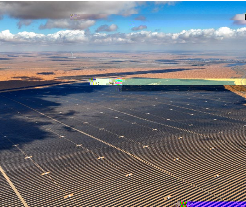
Tengri Desert "Shagehuang" New Energy Base project in Ningxia
